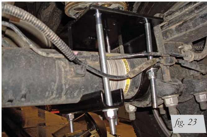
Right side (passenger's) view towards rear of finished installation torqued to 10 lb.-ft. (14Nm).
